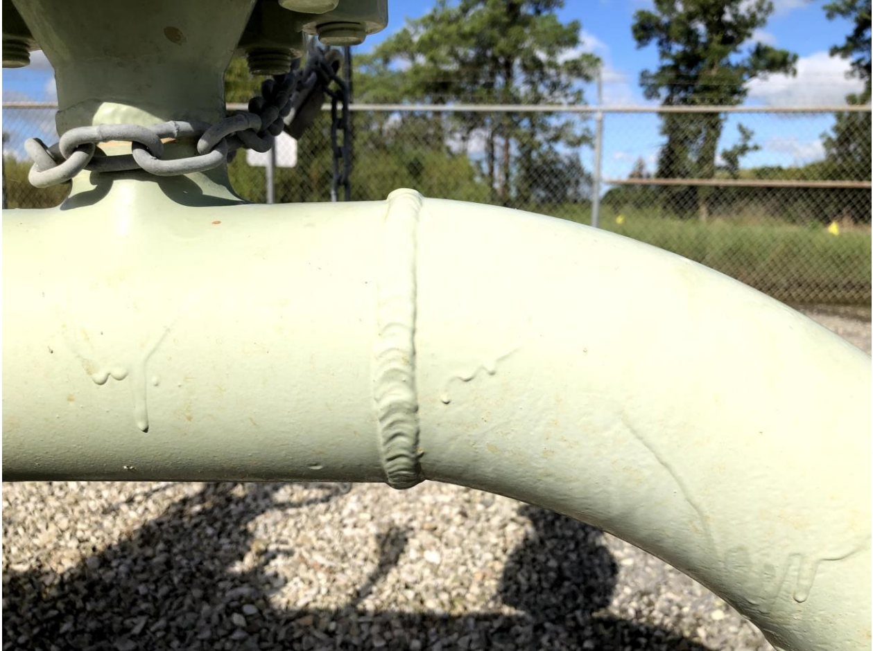
Figure 1 Location of 3.6" Restriction--Sch. 80 Bend and Tee (Note the High/Low Weld)
